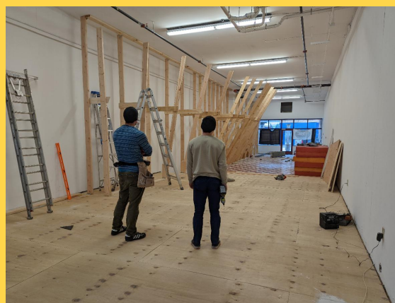
Board members Alex (L) and Tony (R) scrutinize the completed wall framing
